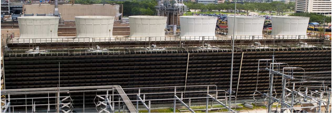
Figure 11.2 A mechanical-draft cooling tower. The fans are located within the cylindrical housings at the top. Air is drawn in through the louvres on the side.
